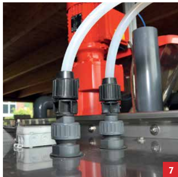
Acid / lye cleaning connection at the mixing tank
