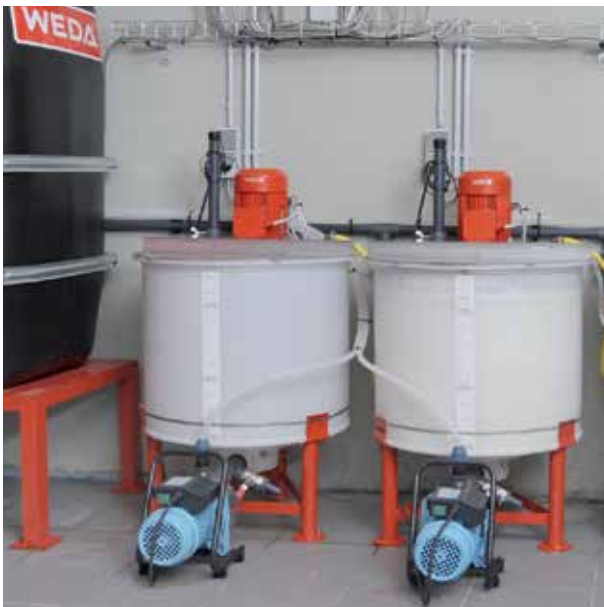
Additive dosing unit
