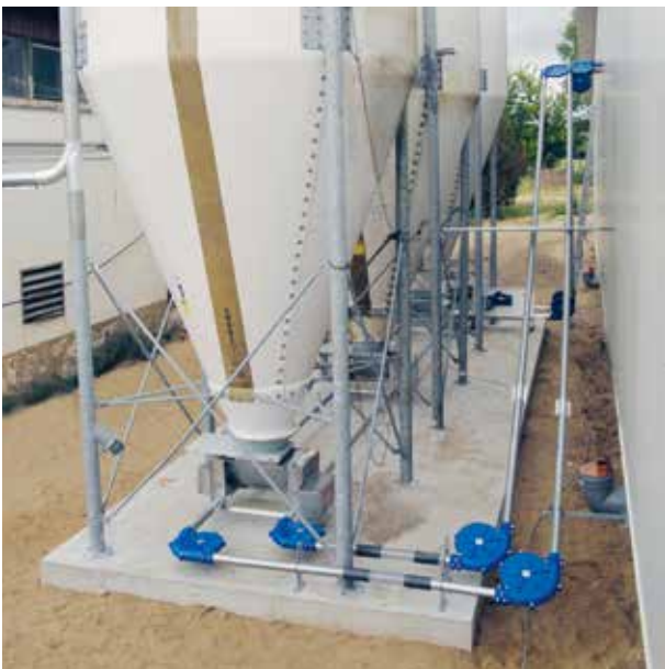
Outdoor silos for dry feeding
