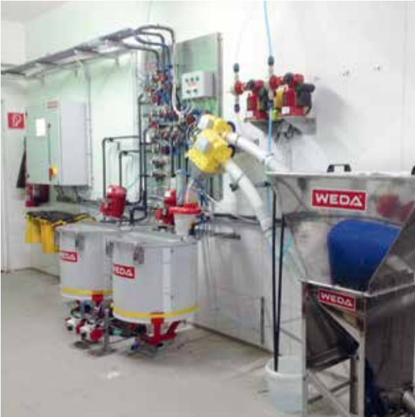
Nutrix with 2 mixing tanks with feed dosage FD
