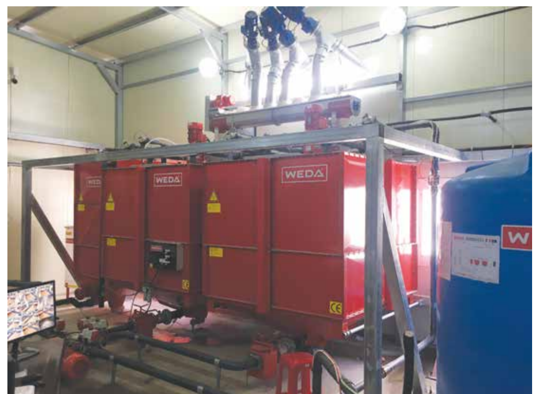
All production areas are supplied with a total of three WEDA liquid feeding systems.
