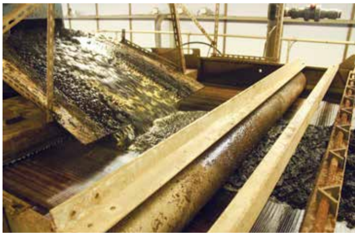
Drainage with belt filter press
