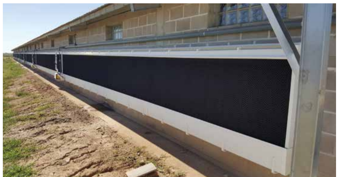
The pad cooling system provides comfortable temperatures in the house.
