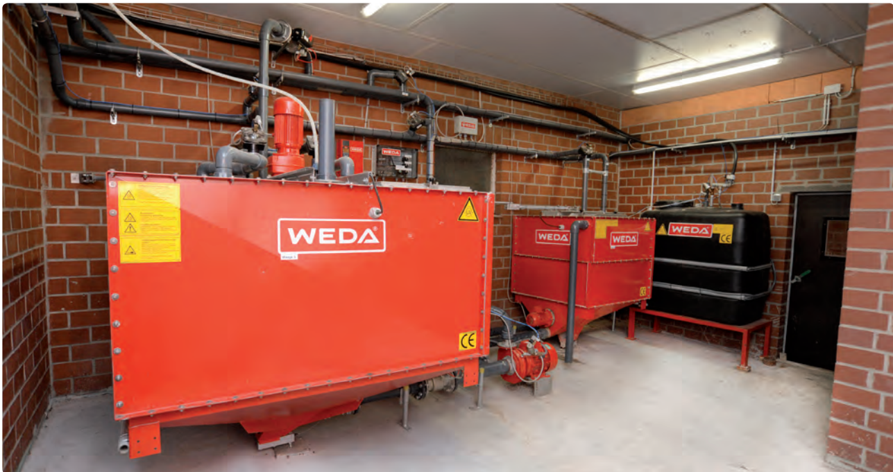
In case of very large distances between feed preparation and animal location, feed provision takes place via satellite preparation room.
