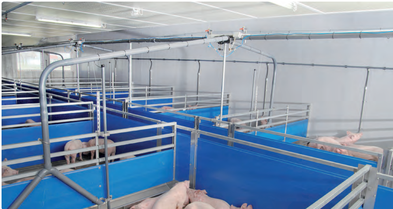
Feed line installed above the walkway.
